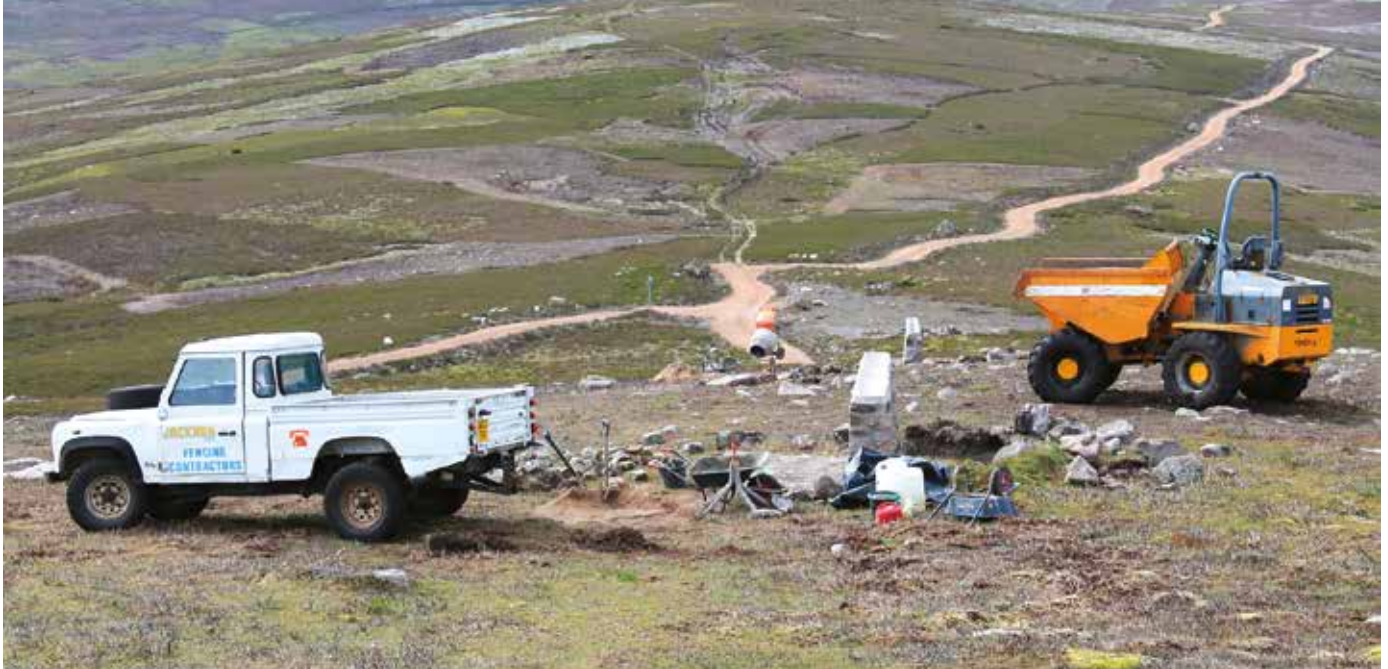
New grouse butt construction with Firmouth and Scottish Rights of Way sign indicating junction between the ancient Firmouth and Fungle routes (Grid Ref. NO499853) Photo: James Carron
