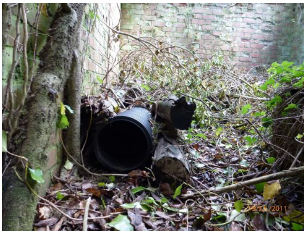
Fig 8: Plastic piping forming an artificial earth above ground near Chipping Norton. In 2003 this artificial earth was built from vehicle tyres, suggesting this new earth was constructed in 2004 or later.
